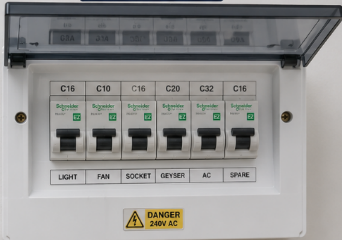
3. MCB FUSE BOX
